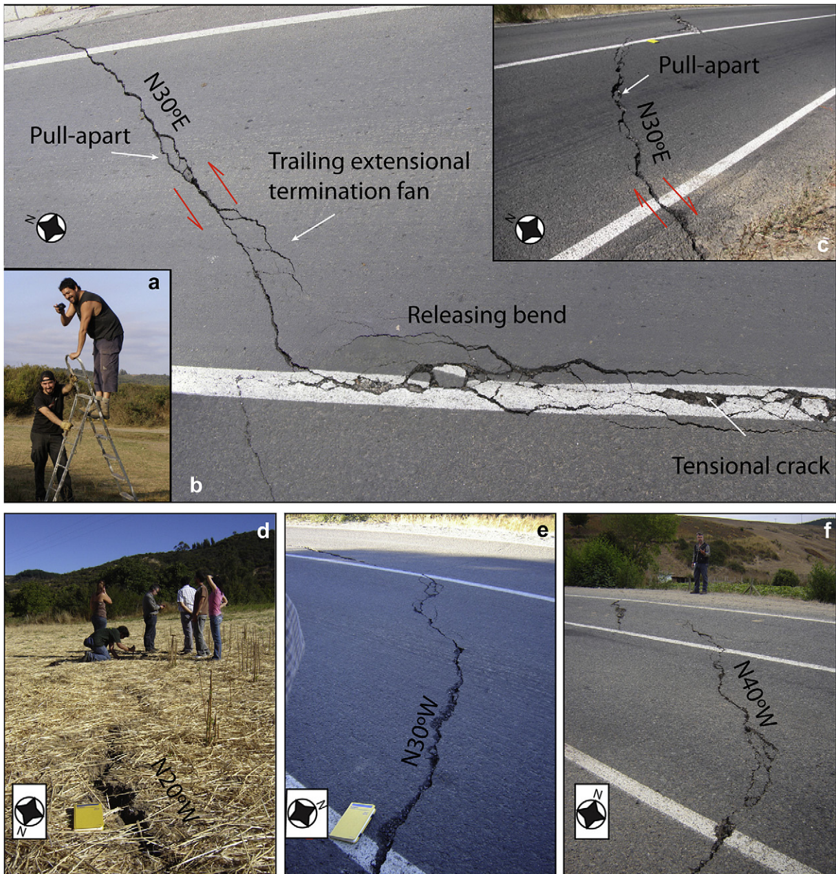
Fig. 2. Representative photographs of co-seismic open cracks without significant vertical displacements. (a) During the field trip a stepladder was used to obtain nearly orthogonal to the surface images in order to map the main structural features; (b) Main structural features draped over a nearly orthogonal photograph showing co-seismic NE-SW left-lateral and normal displacement in locality A. (c) Evidence for NE-SW right lateral and normal displacement in locality A. (d) \text{N}20^{\circ}\text{W} extensional cracks in locality A. (e) Evidence for NW-SE extensional cracks with left-lateral displacement in locality A. (f) NW-SE extensional cracks in locality D.
